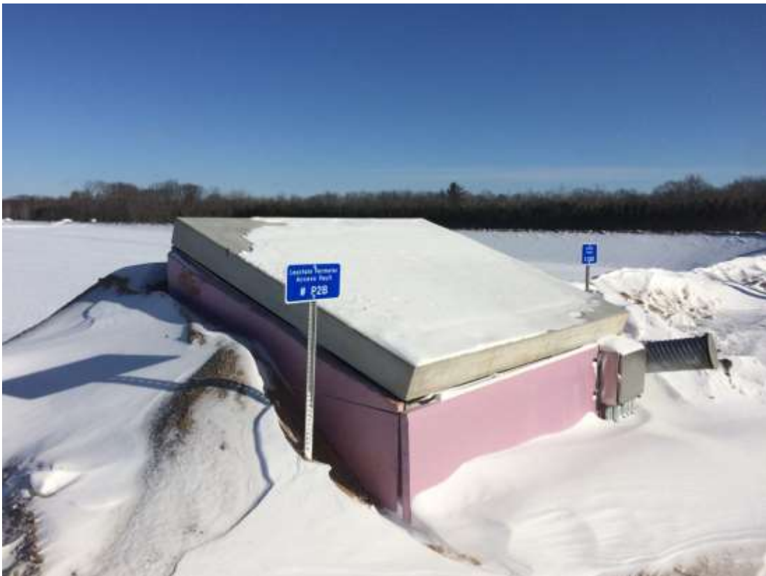
Photo 8 - WDS No. 3 looking Leachate Extraction Vault P2B.
