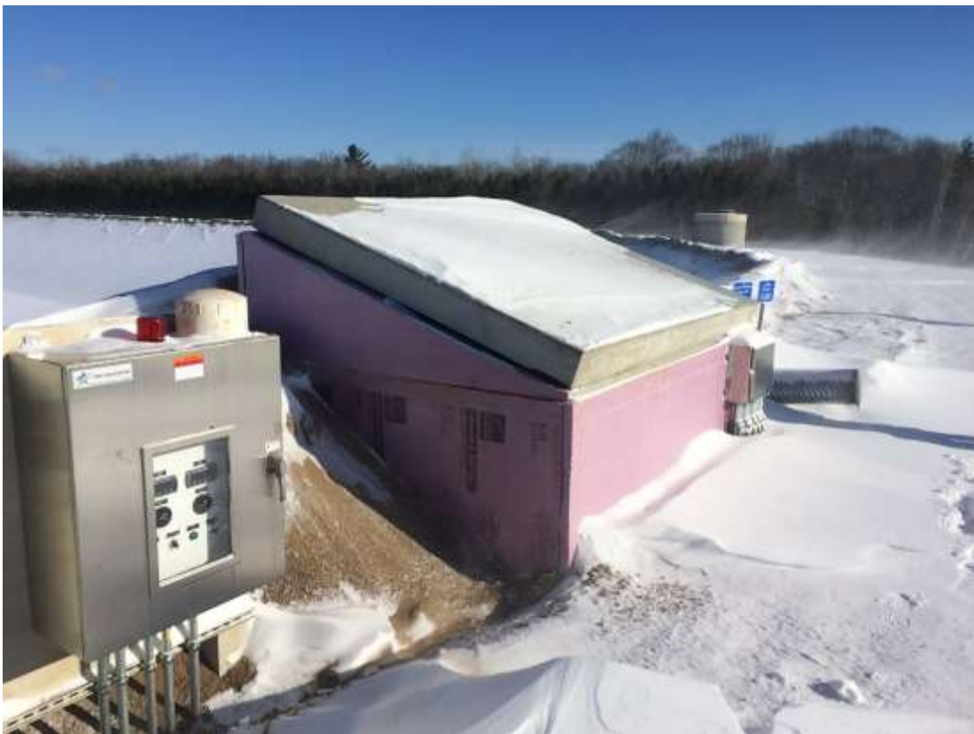
Photo 6 - WDS No. 3 looking at Leachate Extraction Vault P2A.
