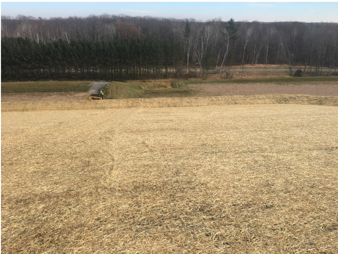
Photo 6 – Looking east from top of Cell 2 partial final cover at Stormwater Basin 2 and 3.
