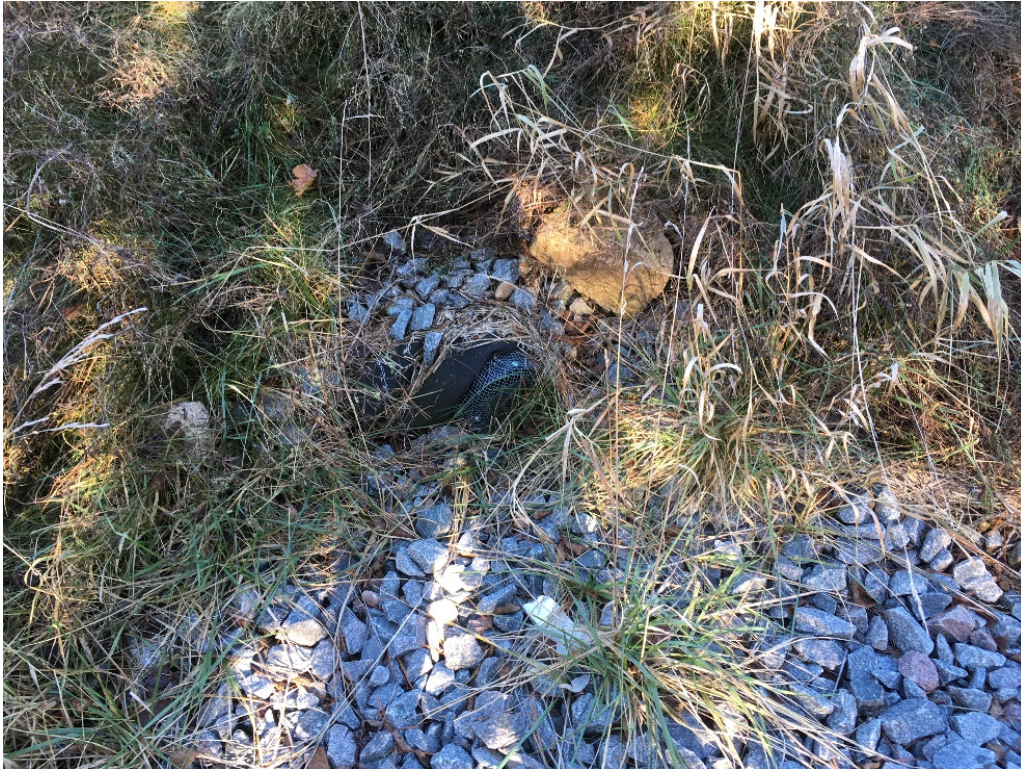
Photo 2 - Gradient control pipe slightly east of westernmost gradient control pipe along south perimeter berm
