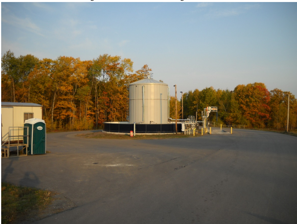
Photo 12 – Leachate collection tank and loadout facility.
