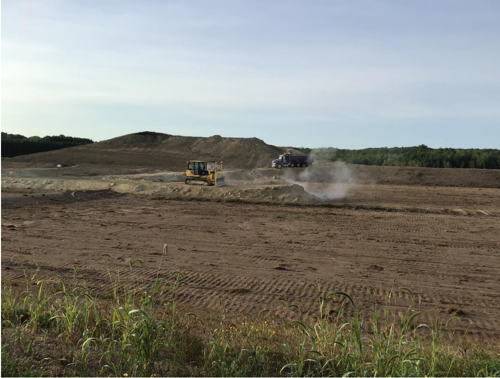
Photo 7 – Placing and spreading the frost protection layer in August. Vegetation was stripped before placement.
