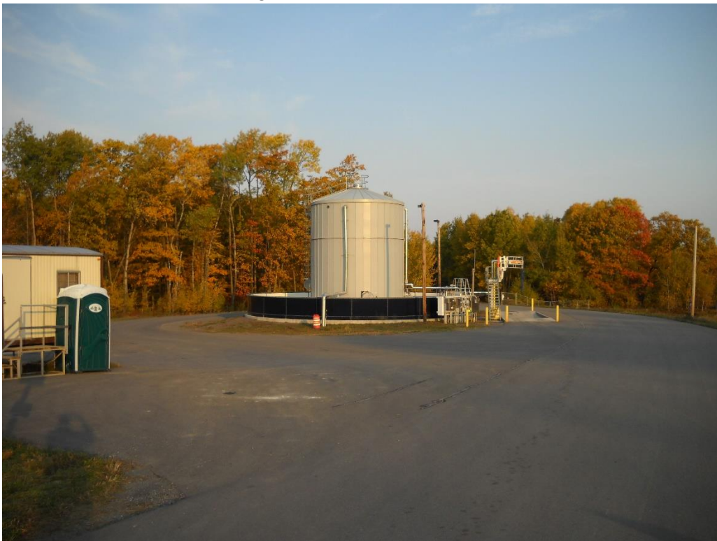
Photo 12 – Leachate collection tank and loadout facility.
