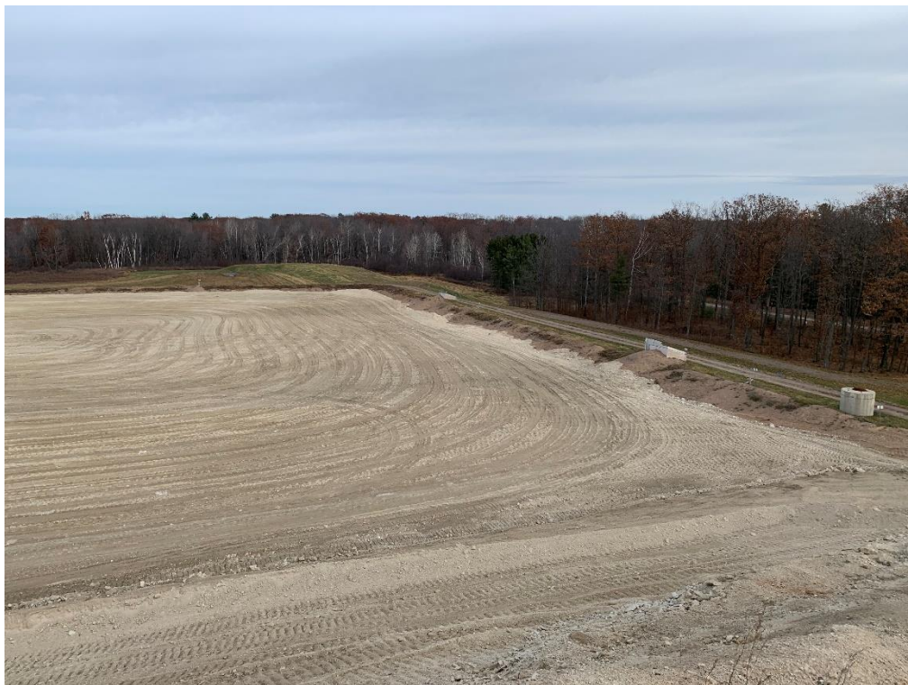
Photo 8 – Looking north to the Cell 1 active filling area showing frost protection layer.
