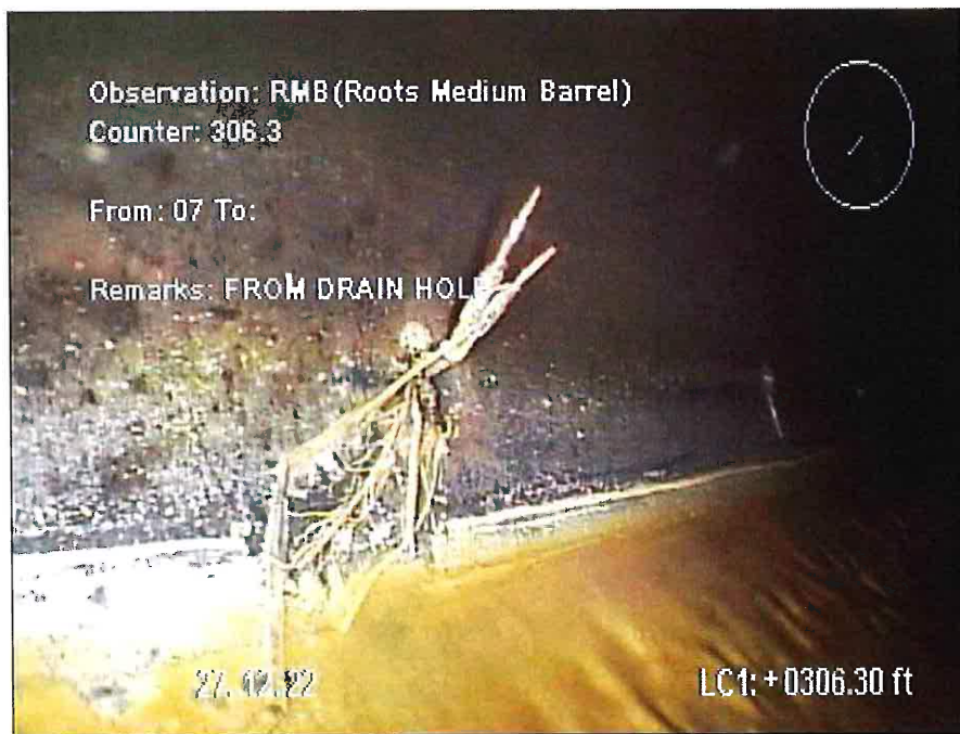
Date: 2022/12/27 Distance: 306.3 Ft Obs: Roots Medium Barrel Comments: AT DRAIN HOLE
