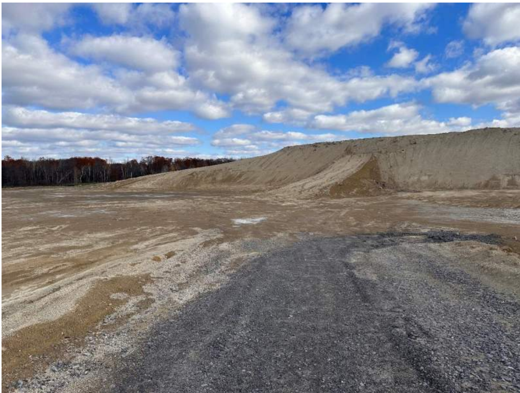
Photo No. 10 – Looking northeast to the Cell 1 active filling area and east slope.
