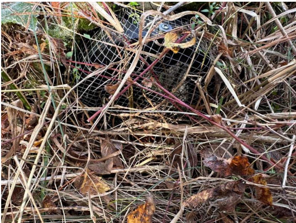
Photo No. 14 – Cell 2 gradient control outlet pipe.
