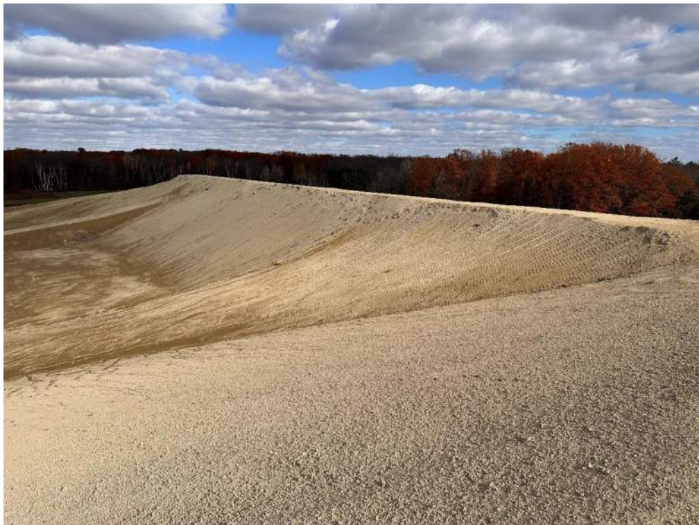
Photo No. 8 – Looking northeast to the Cell 1 active filling area and the east slope prepared for final cover.
