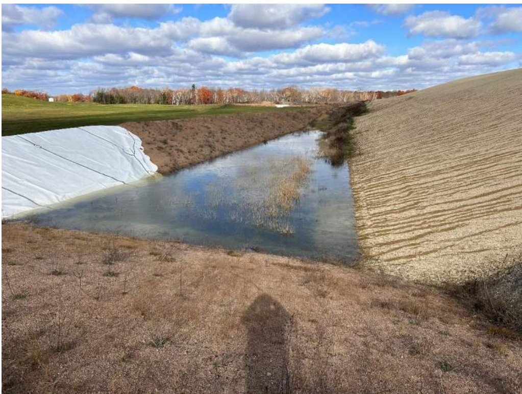
Photo No. 2 – Cell 2/3 intercell berm and leachate collection ditch along west side of Cell 2.
