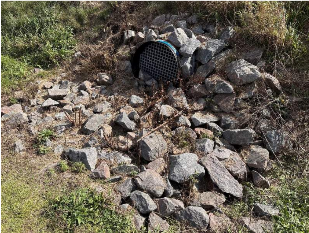
Photo No. 13 – Stormwater diversion berm inlet on the southeast corner of Cell 2.
