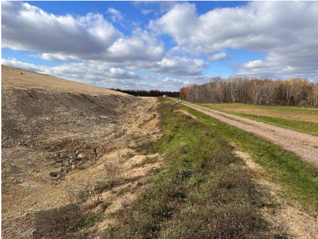
Photo No. 9 – Looking west at the Cell 1 north perimeter slope and leachate collection ditch.
