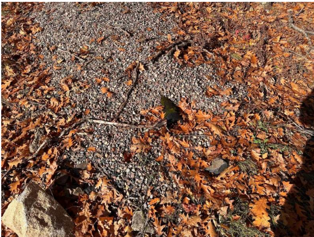
Photo No. 16 – Cell 1 gradient control outlet pipe.
