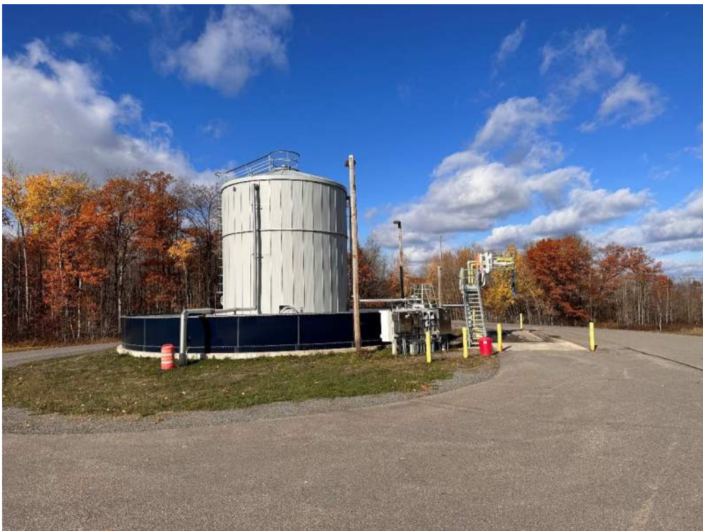
Photo No. 12 – Leachate collection tank and loadout facility.
