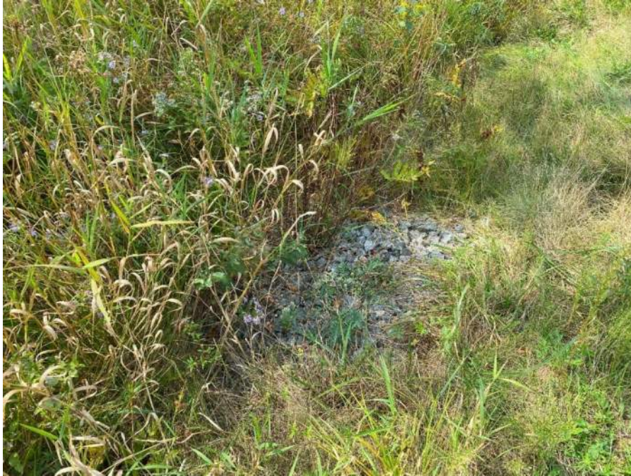
Photo No. 13 – Cell 2 gradient control outlet pipe.
