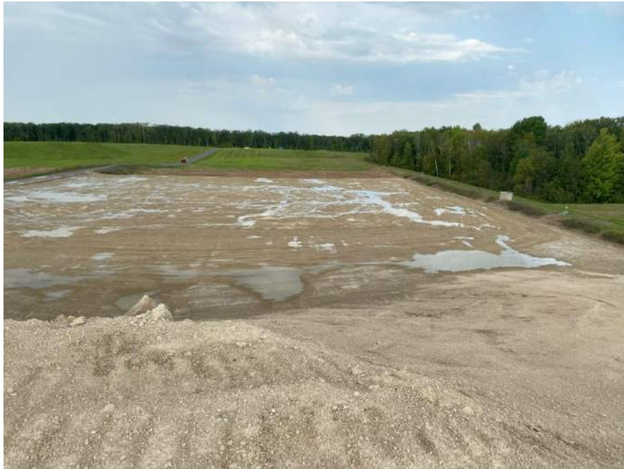
Photo No. 7 – Active filling area in Cell 1, looking west. Active area watered for dust control.
