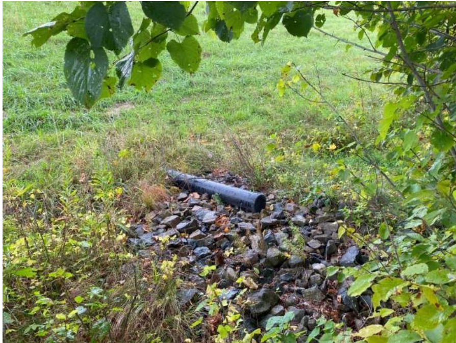
Photo No. 15 – Cell 1 gradient control outlet pipe.
