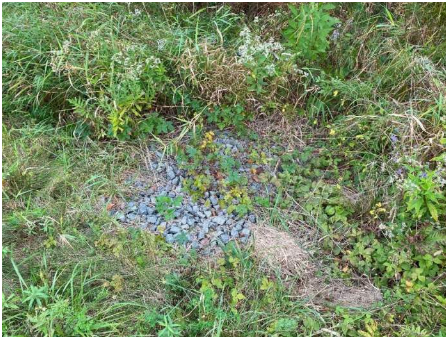
Photo No. 14 – Cell 2 gradient control outlet pipe.
